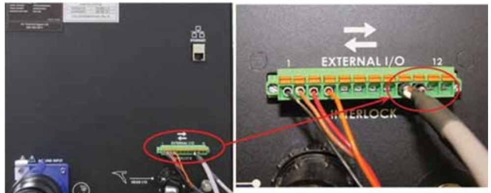
Figure 30: Connect the Synch Cable Wires to the 12-pin I/O Connector
